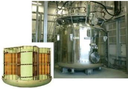
Figure 2. 10 MVA/1 s SMES at Kameyama field test, in Japan. Image from [4].
