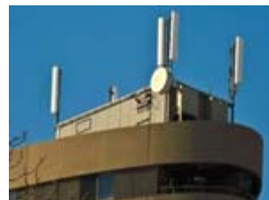
“Roof top” radio site
